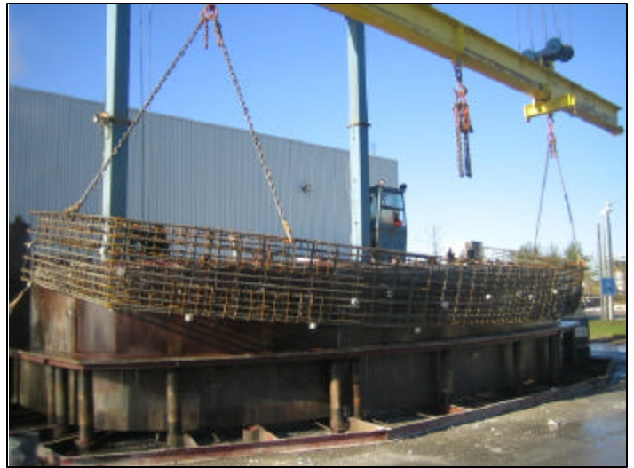
Placement of rebar cage in mold with a span of 10.98m and vertical rise of 3.96m.
